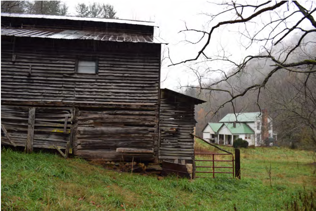
Southwest (side) elevation of the livestock barn with view to the house, view to the east-northeast
